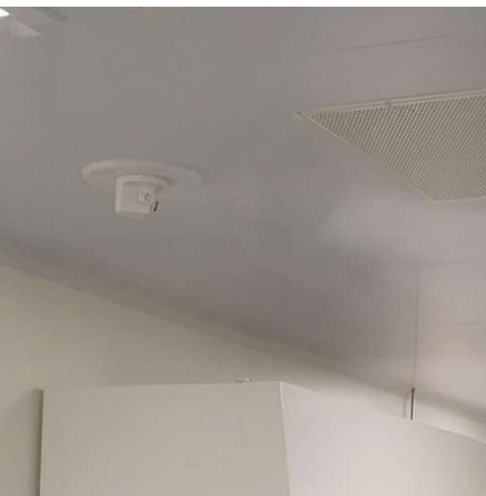
Remote Spray Head installed in cleanroom ceiling
